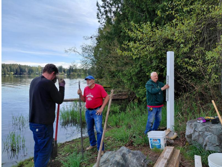
On 18 April 2026 Barry, Frank, Jim, & Carl installed the signposts for the Boat Launch Safety Sign at the DFW Boat Launch.
