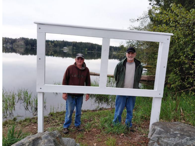
On 20 April 2026 Barry and Curt installed the sign frame for the Boat Launch Safety Sign at the DFW Boat Launch.
