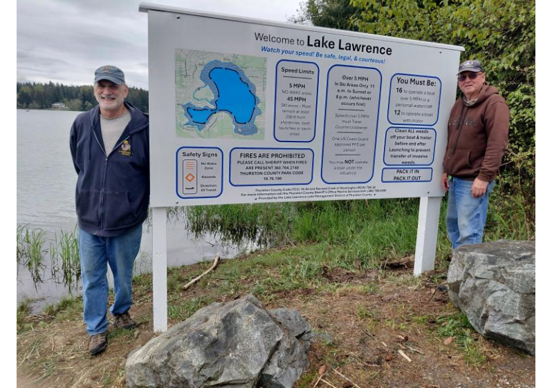
On 21 April 2026 Barry and Curt installed the sign for the Boat Launch Safety Sign at the DFW Boat Launch.
